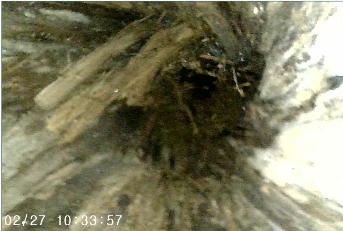
PHOTO 1-7: INTERIOR OF THE CAVITY AT SITE JBL-1205-001 SHOWING EXTENSIVE DECAY
