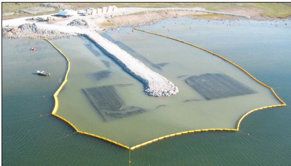
Plate 5.12-2. Example of a turbidity curtain used for the construction of a jetty.
