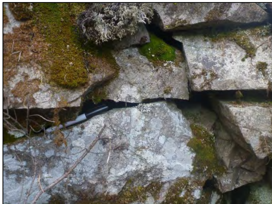
Photo 14: Crevice observed at 117lo
