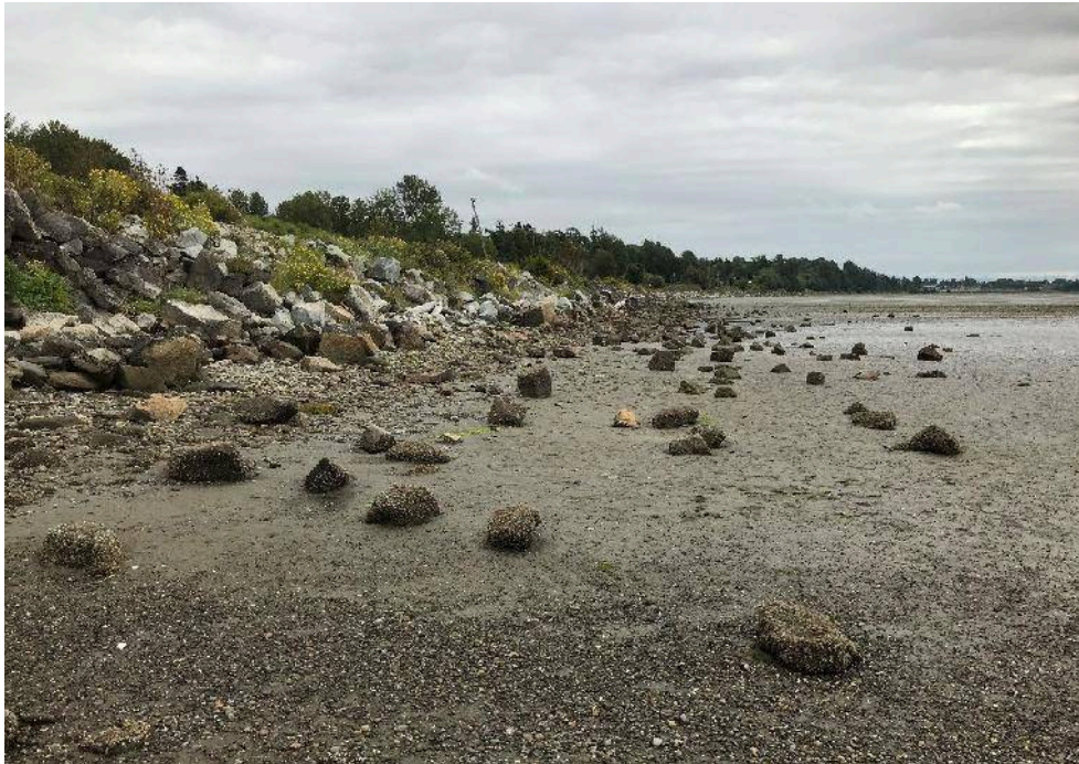
Photo 3.3 Relatively deflated beach profile with fine sediments extending up to the base of the existing riprap slope, on the southeast side of the river mouth (looking southeast)
