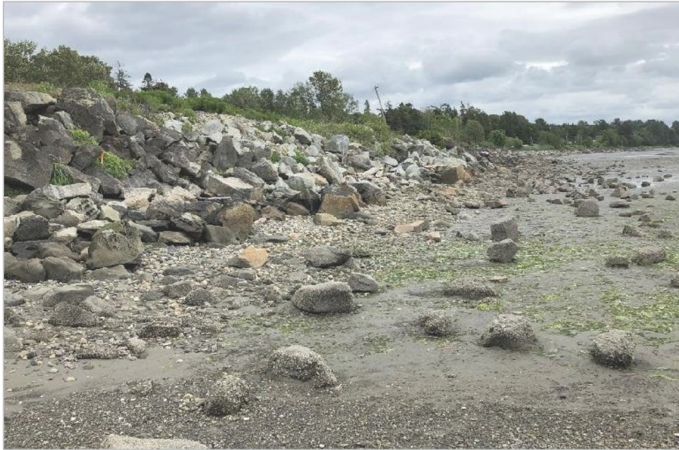
Figure 13: East View of Eastern Semiahmoo Bay Foreshore Area Targeted for Groyne Implementation and Sandy Gravel Beach Enhancement as part of the Semiahmoo Project (Taken May 22, 2020)
