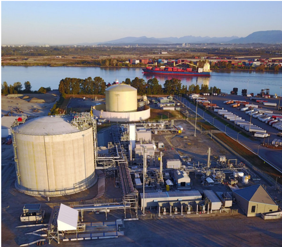
Photograph 1: View of Tilbury facility with new storage tank in foreground, and original tank in the background.
